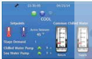
Select chilled water temperature setpoint and cool/heat modes in main control screen
