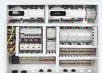
Enclosure interior features circuit breakers for compressors and pumps; circuit boards are coated for corrosion resistance
