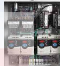
Custom-made fan control enclosure with VFDS
