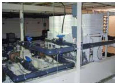
Cruisair three-stage chiller on-board Lady of the Lake
