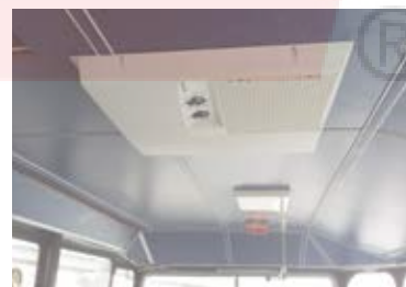
The DuraSea Air Distribution Box with controls and return air in the pilot-house of the Bahamas Ferries Sealink catamaran.
